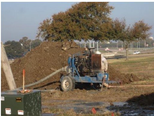
Slurry Return Pump
