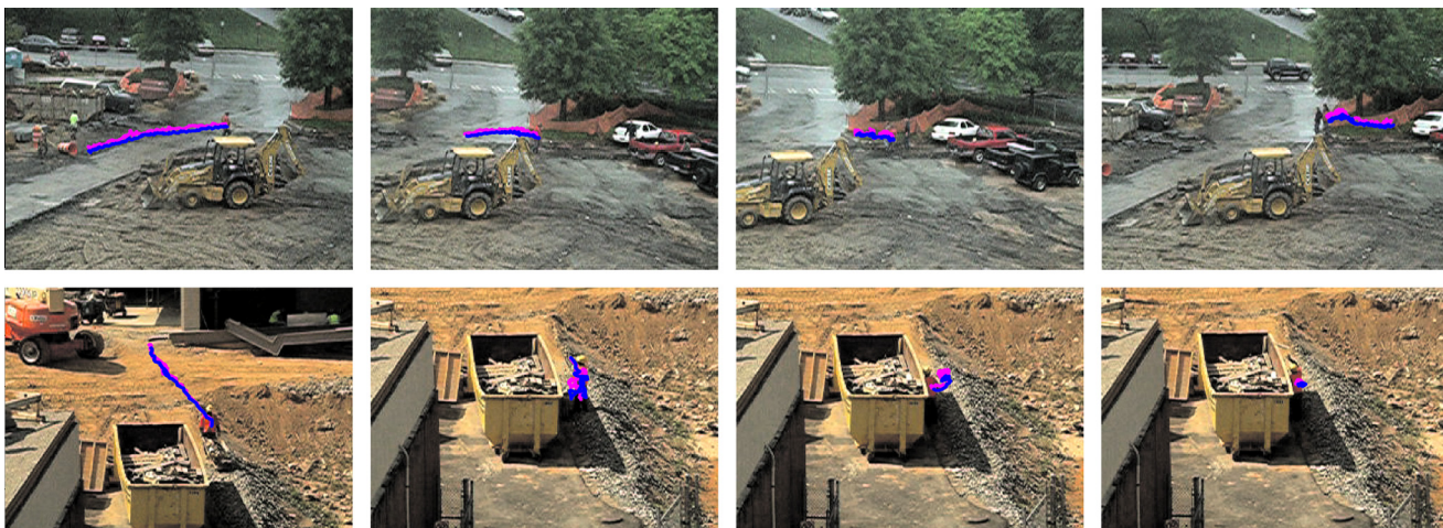
Fig. 5. PTZ camera tracking: Following a construction worker using mean-shift (magenta) and Bayesian segmentation (blue) [89]. (For interpretation of the references to color in this figure legend, the reader is referred to the web version of this article.)
