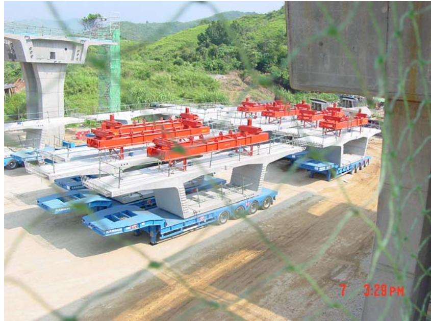
Figure 4.2: Bulky Precast Segments (12m x 2.5m x 2.8m Each) Temporarily Stored around the Working Span
