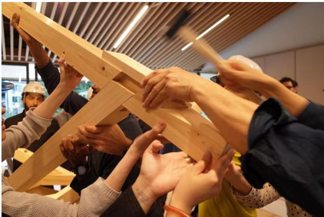
Figure 9. The assembly of the Pagoda exemplified the elegance (and challenge) of joint connections that avoided the use of fasteners between the timber elements.
