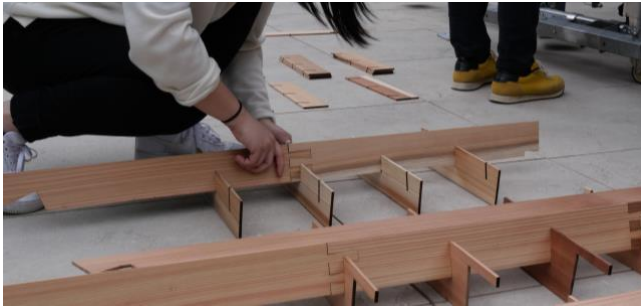
Figure 11. The roof of the Pagoda took full advantage of the laser cutter, in which all pieces were cut and labelled for pre-assembly before connecting to the structure.
