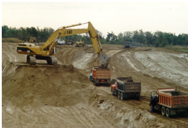
Fig. 2 In a road projects, multiple clients (haulers) form a queue in front of a single processor (excavator).
